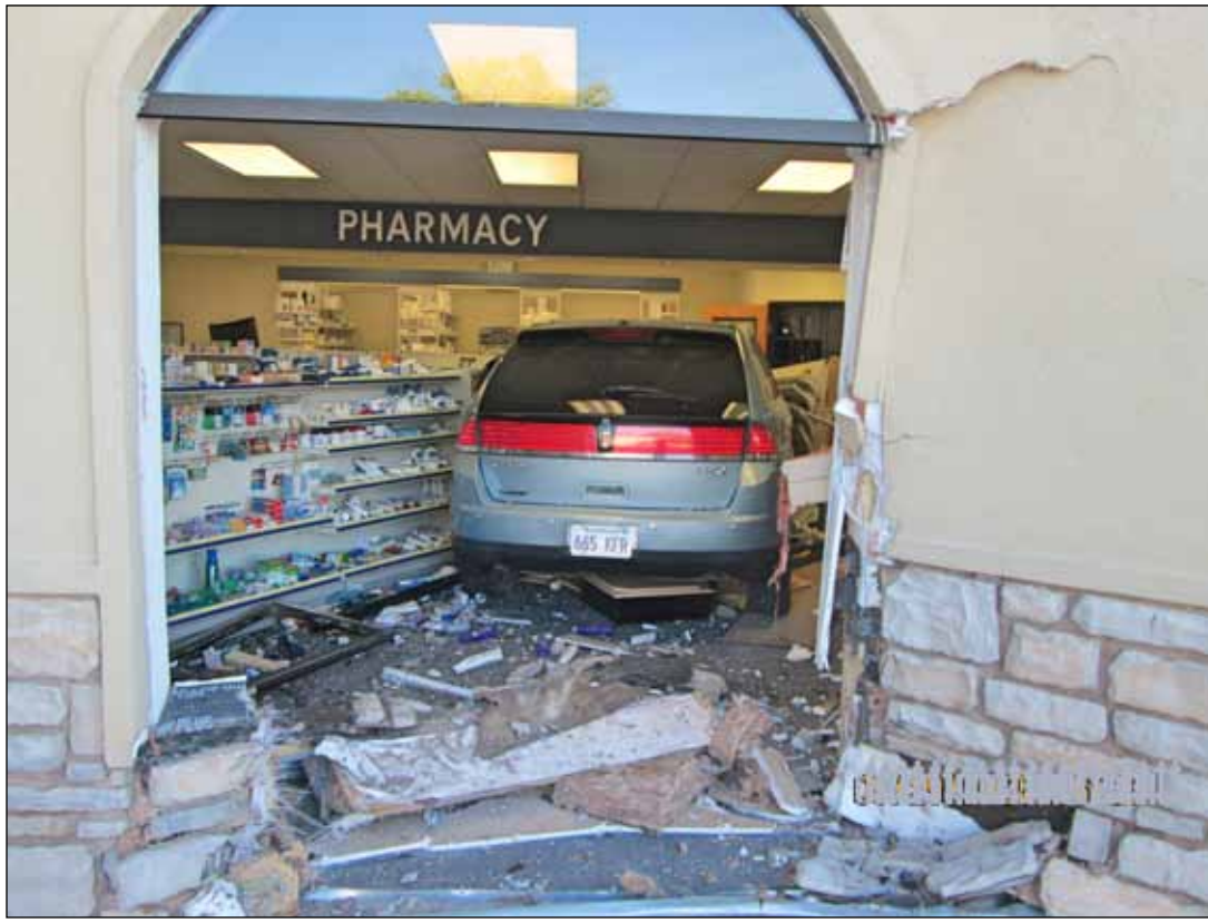
The aftermath of an accident where a car drove through the front of The Medicine Shoppe on Sept. 29.
